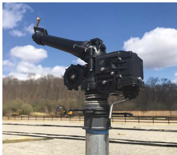
Turbina ST-1200-BR installata
